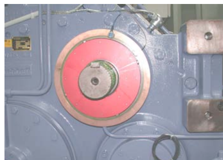
Rotor und stator (antenna) on the high speed shaft of the gearbox.
