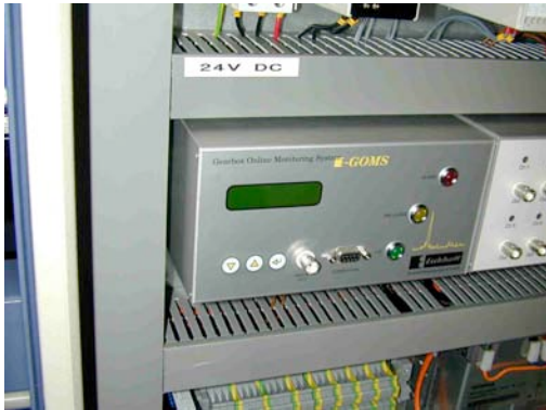
E-GOMS I vibration monitor
